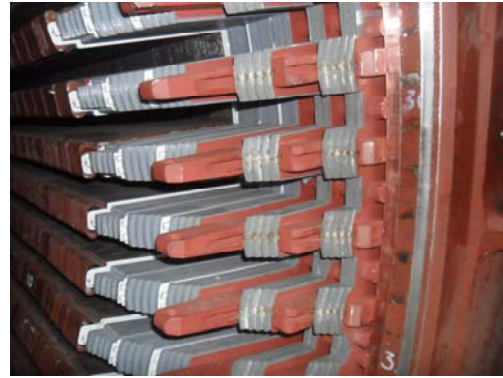
Figure 3. Modernized end part of the magnetic stator core of turbo-generator n.1 in TPP Bitola
